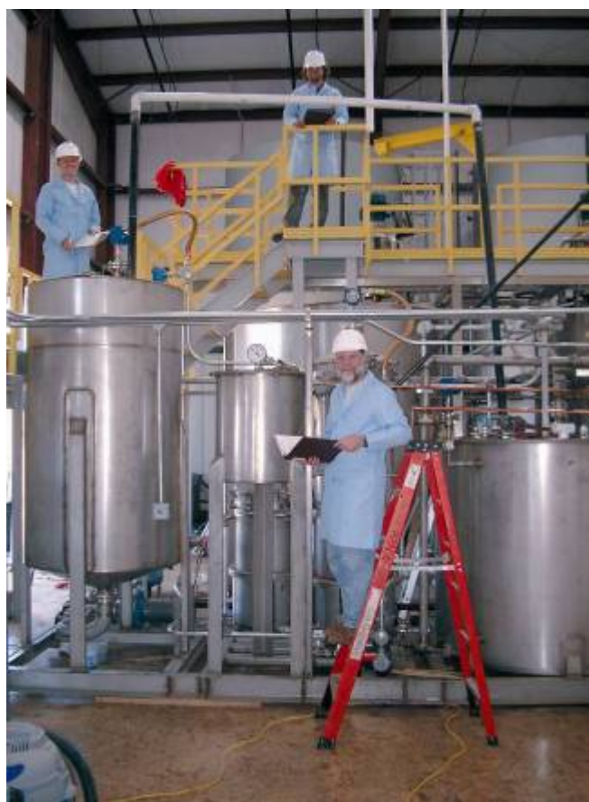
MPU installed and in operation at Denton, Texas
